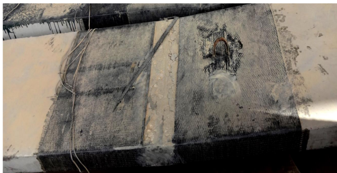
Fig. 24. Girder RGR concrete slab crushing at the mid-span
